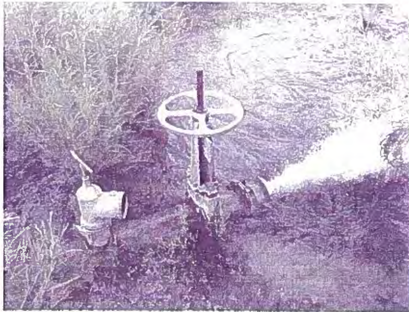
This is the outlet of the 8" penstock. The water currently flows into the Kingston Creek Ditch and into the Young Brothers Reservoir. The water is used for irrigation.
